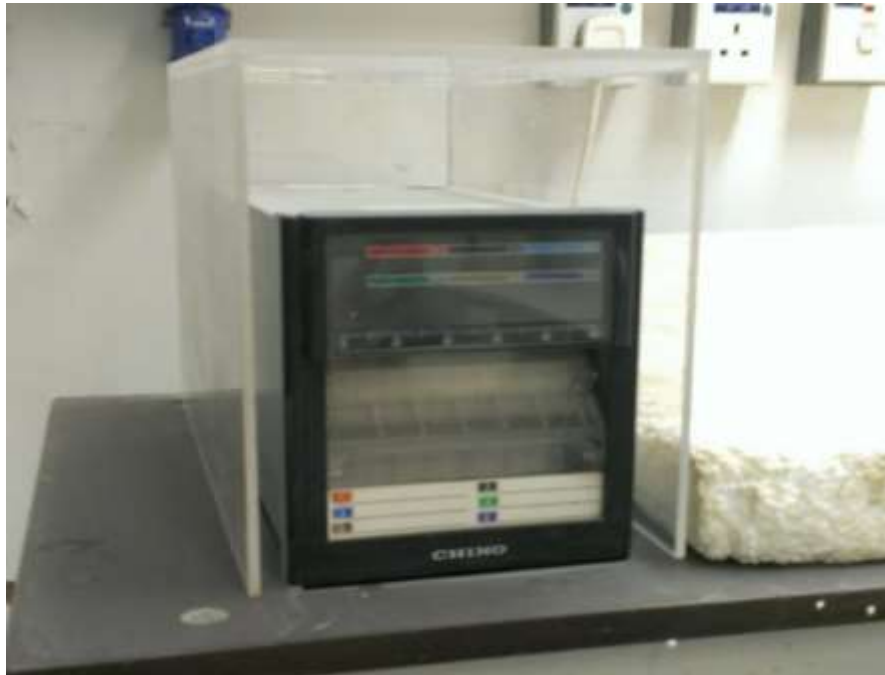
Picture 2.3.3.2-Temperature control unit of the water tanks
